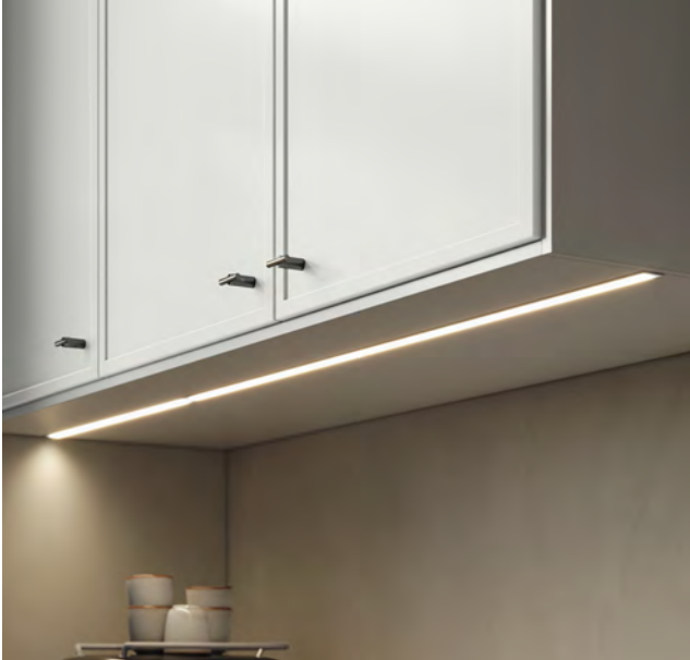
Lighting strip under wall cabinet
